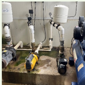
2 Vacuum pumps with no VSD above and left (e.g. there are no wires connecting to a control box). Distinctive vacuum cylinders (in white above) and wide pipes identify the vacuum pump.
