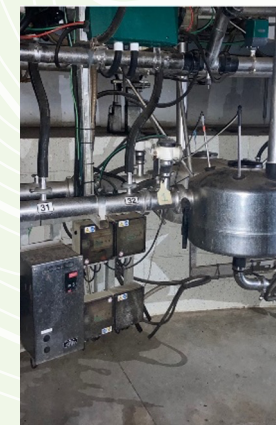
4 Rotary drive in the pit with VSD (see arrow)
