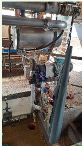
Vacuum pump on the right has cables from pump to the VSD.
